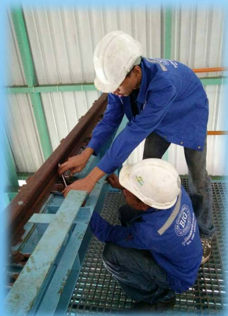
Services overhead crane
