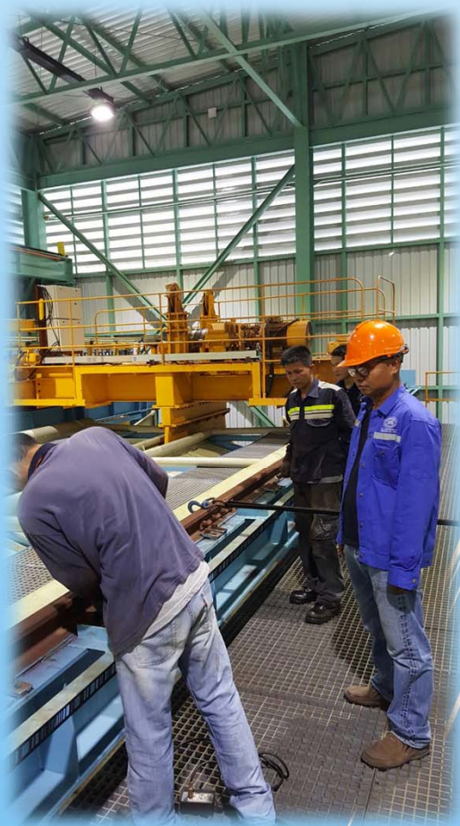
Services overhead crane
