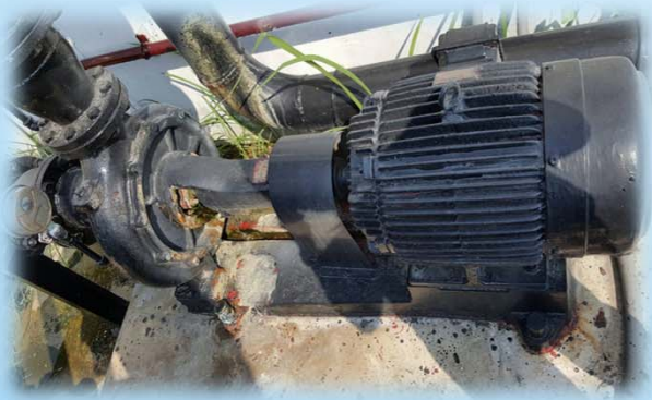
Cooling motor pump
